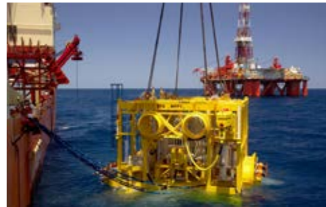
Installation of a OneSubsea Dual Pump Station (Source: OneSubsea)
